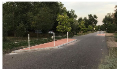
Installed a chicane on Upland Avenue as a pilot—innovation in both traffic calming design as well as project delivery
