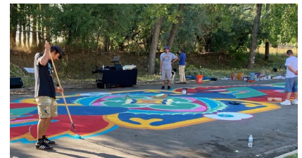
Worked with Boulder Arts and StreetWise to deliver a street mural as a traffic calming experiment on 34th Street in the San Juan del Centro neighborhood, as part of a study for a CU-Denver Masters in Urban and Regional Planning (MURP) capstone project
