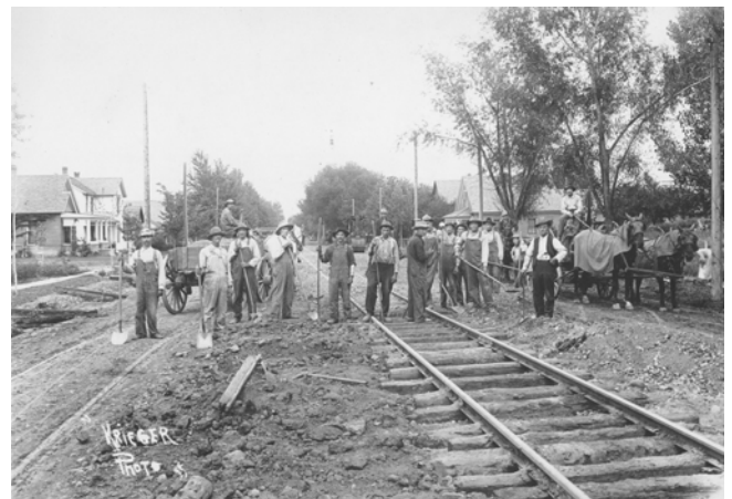
Figure 11 - Work crew lays track for the new streetcars. Krieger photo, A.A. Paddock Collection.
