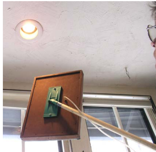
Figure 2-17. An auditor prepares to assess a recessed lighting fixture on the 1 st story of a 3rd story house for air leakage (with the blower door running.) It was quite leaky.
