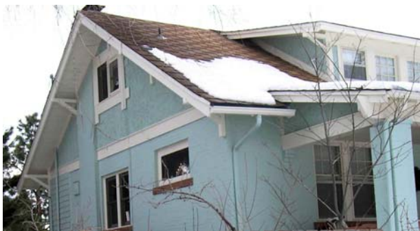
Figure 2-3. Snow on the roof of this historic house suggests a lack of insulation toward the peak of the roof.
