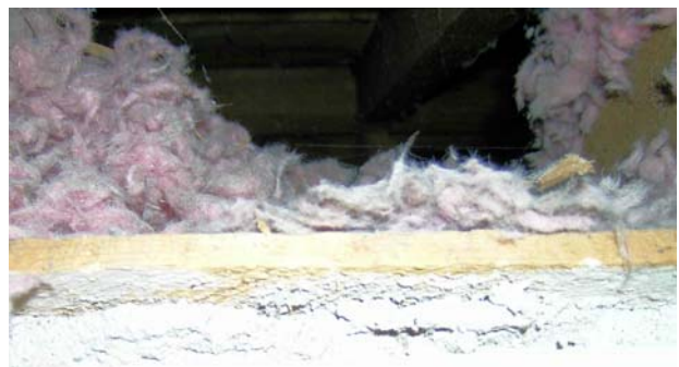
Figure 2-4. Sure enough, insulation under the rooftop is less than an inch thick.
