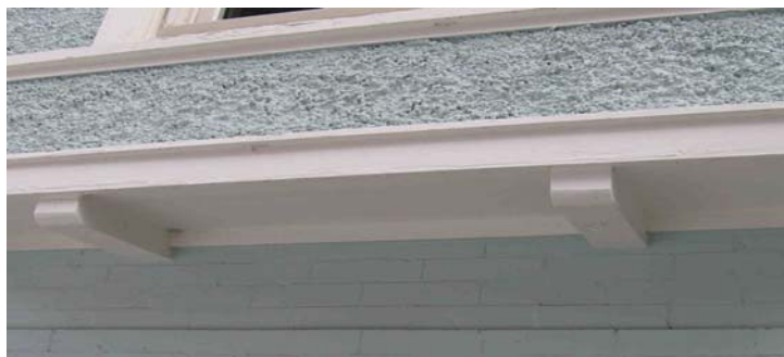
Figure 2-7. Areas like this that protrude from under windows are frequently sources of air leakage and are rarely insulated.
