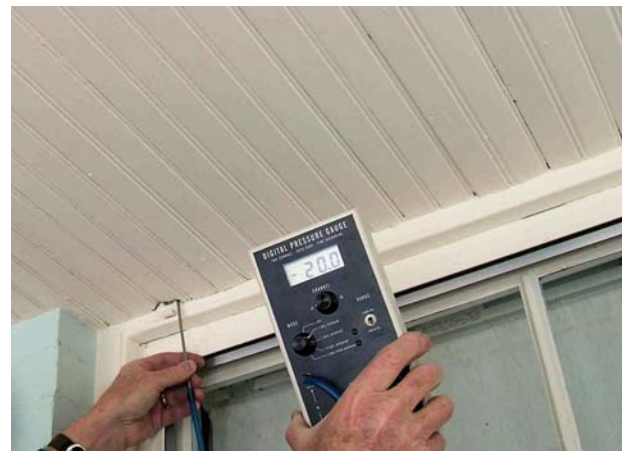
Figure 2-8. Measuring pressure differences between the outside and the cavity above the ceiling of this large porch while the blower door was running showed that the porch is thermally connected to the home's envelope. Blowing cellulose to high density in the cavities closest to the exterior wall will stop the flow of air, save energy, and increase comfort in the bedrooms above
