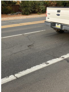
Pothole near Iris Avenue at 26th Street intersection
