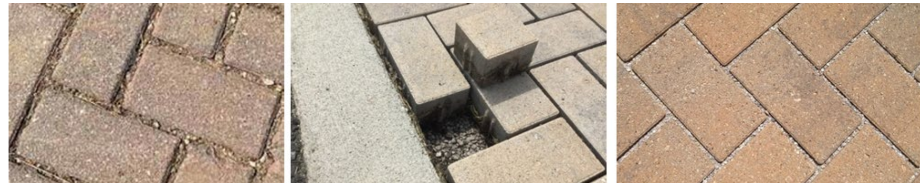
Clogged Joints, Empty Joints and Finished Joints (left to right)
