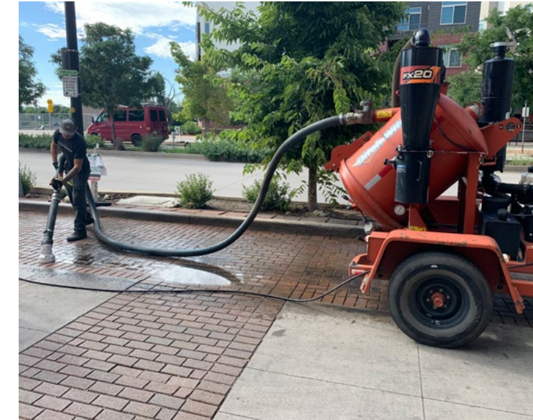
Using a pressure washer with a Ditch Witch FX20 Vacuum to dislodge material from the joint spaces.
