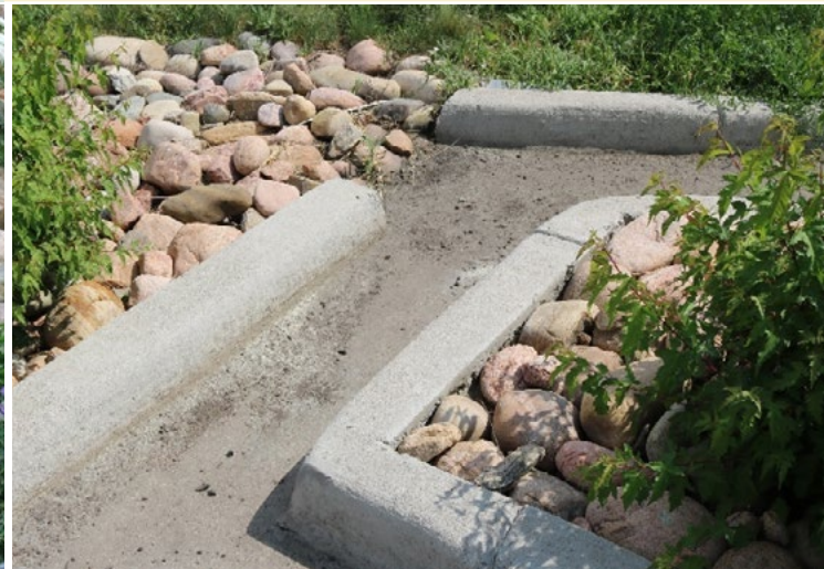
The inlet has sediment buildup, which could prevent the SCM from draining properly. The sediment should be removed with a shovel and disposed of.
