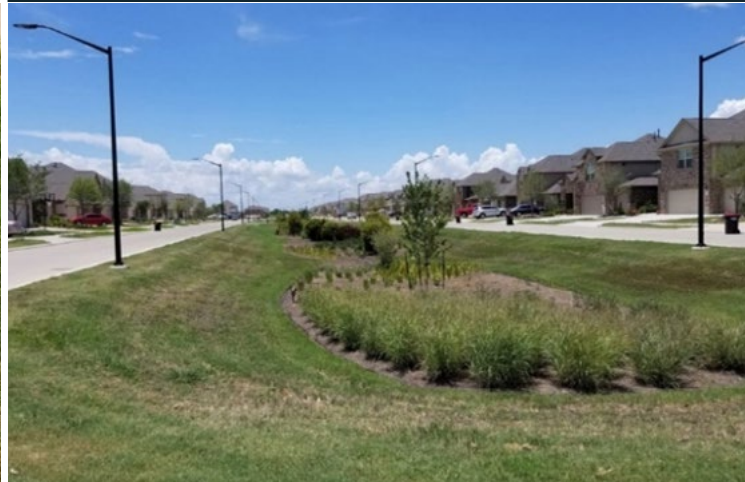
While there are no signs of vehicle or pedestrian traffic, adding informational signs about the bioretention area could help protect the SCM from intrusion and damage.
