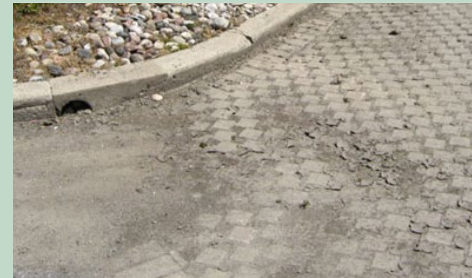
DO NOT neglect maintenance efforts and let sediment build up
