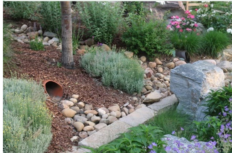
The inlet of this bioretention area is clean and free of debris, allowing runoff to enter the main treatment area.
