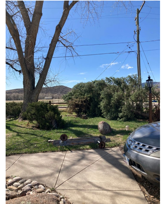
Tree impact with service and cross-arm La Porte, CO
