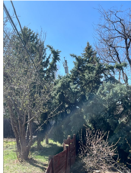
Tree Impact with distribution line Littleton, CO
