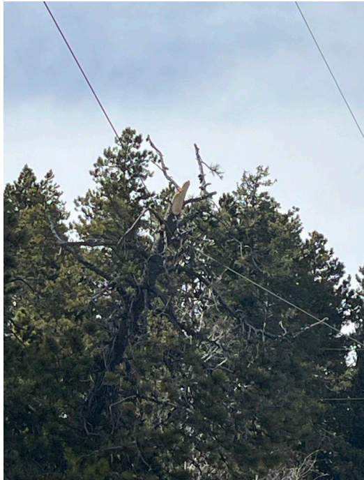
Tree branch breakage in distribution line Boulder, CO
