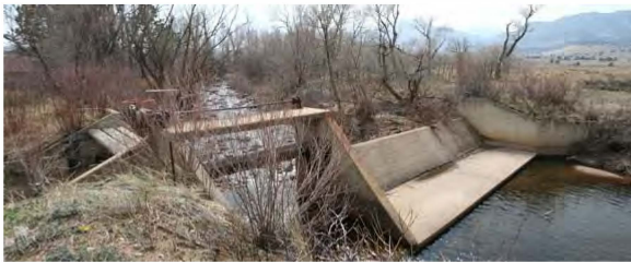
Ditch Diversion a Barrier to Fish Passage
