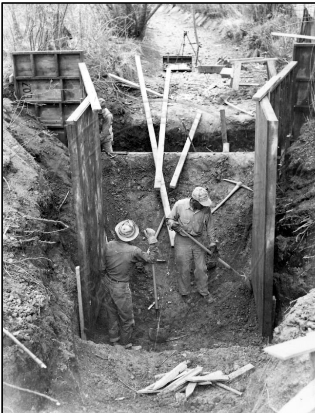
CONSTRUCTION OF THE FARMERS DITCH SIPHON UNDER NORTH BOULDER PARK (1953). SOURCE: CARNEGIE BRANCH LIBRARY FOR LOCAL HISTORY/BOULDER HISTORICAL SOCIETY COLLECTION.
