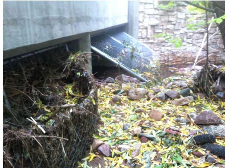
Sept. 2013 Flood Damage
