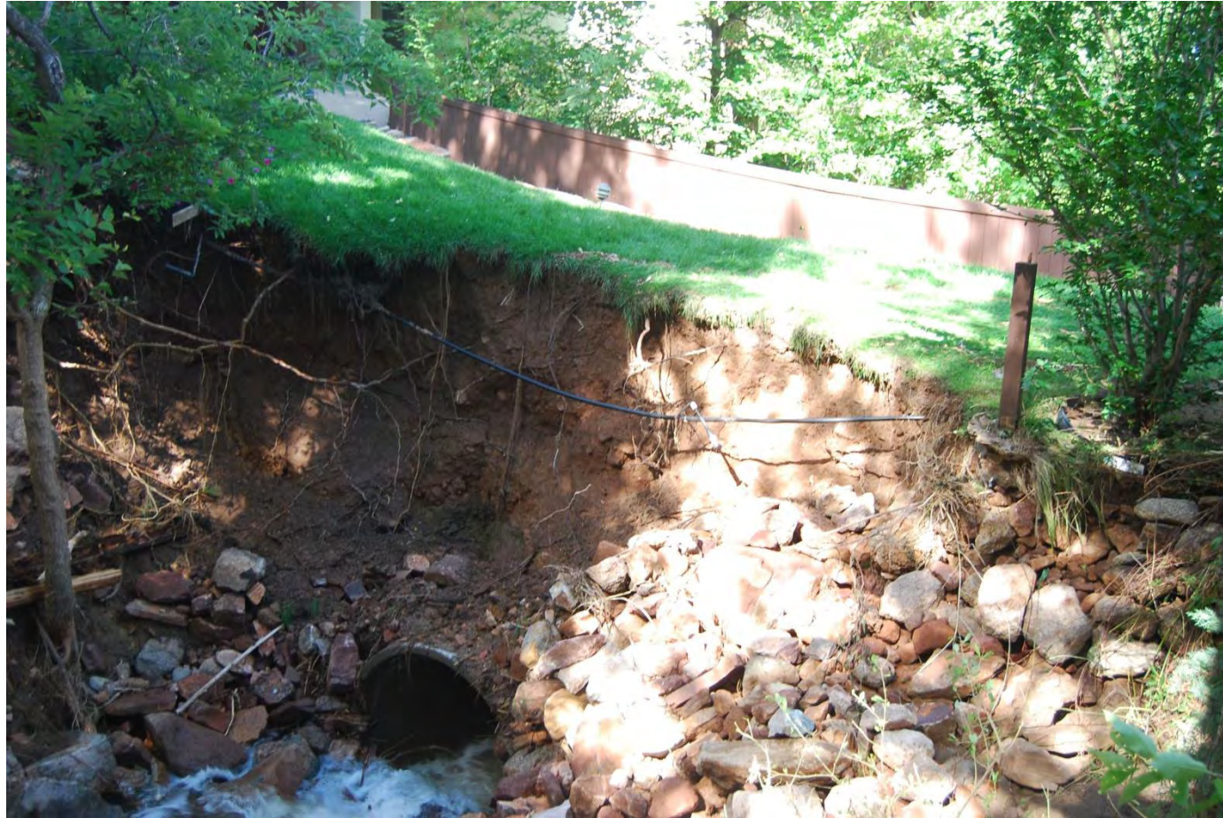
Sept. 2013 Flood Damage
