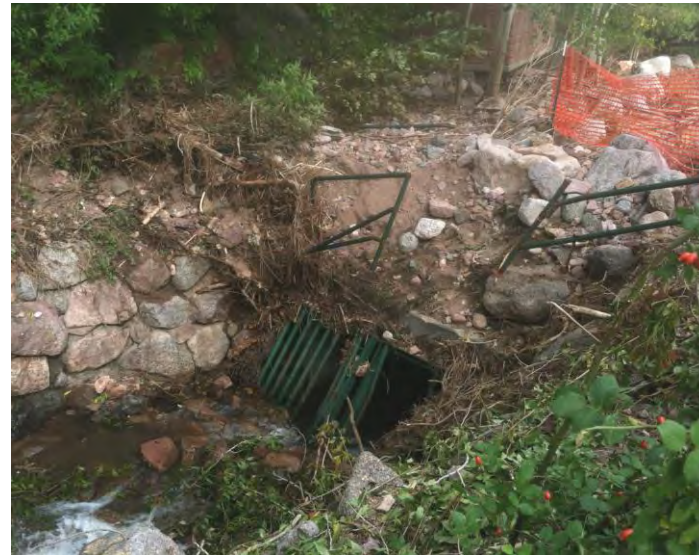
Sept. 2013 Flood Damage
