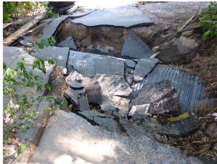
Pennsylvania Ave. Flood Damage
