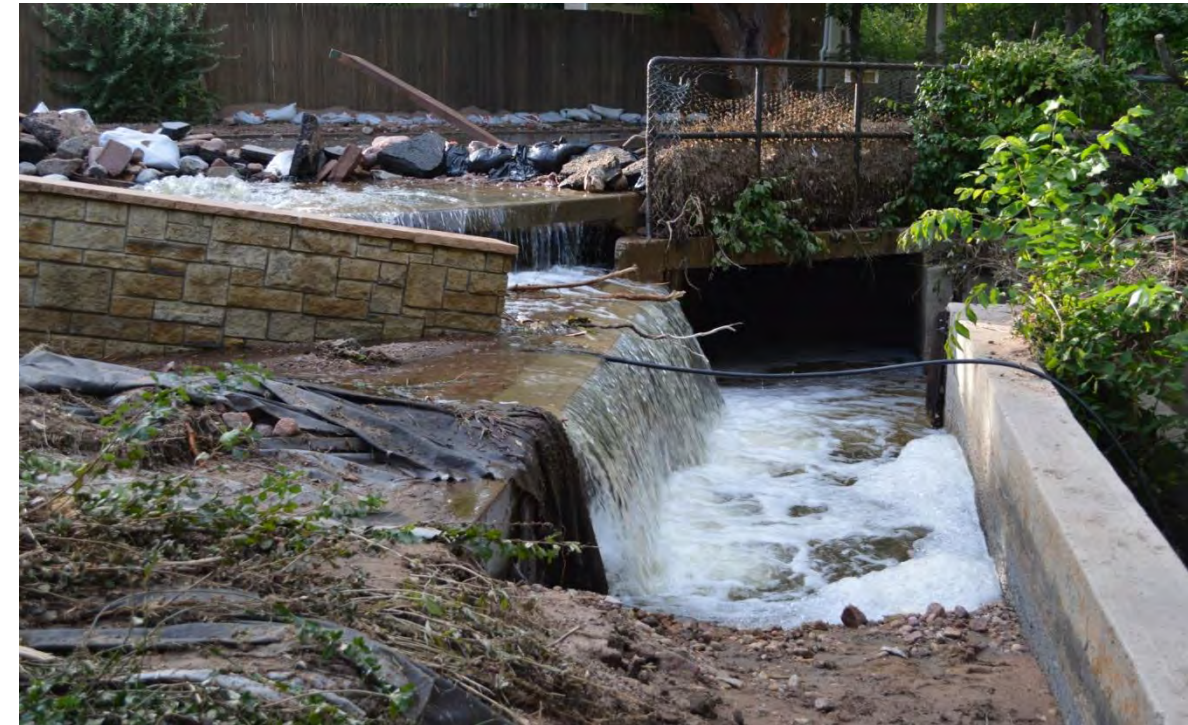
Sept. 2013 Flood Damage (7 th St. and Anderson Ditch)
