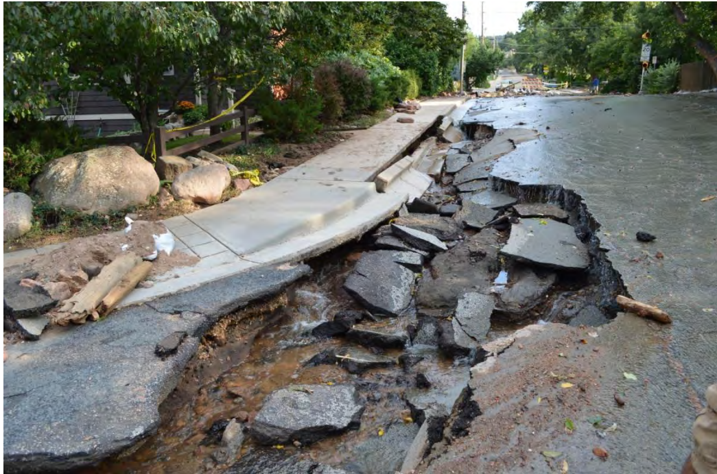
Sept. 2013 Flood Damage at 7 th St. and Pleasant St.
