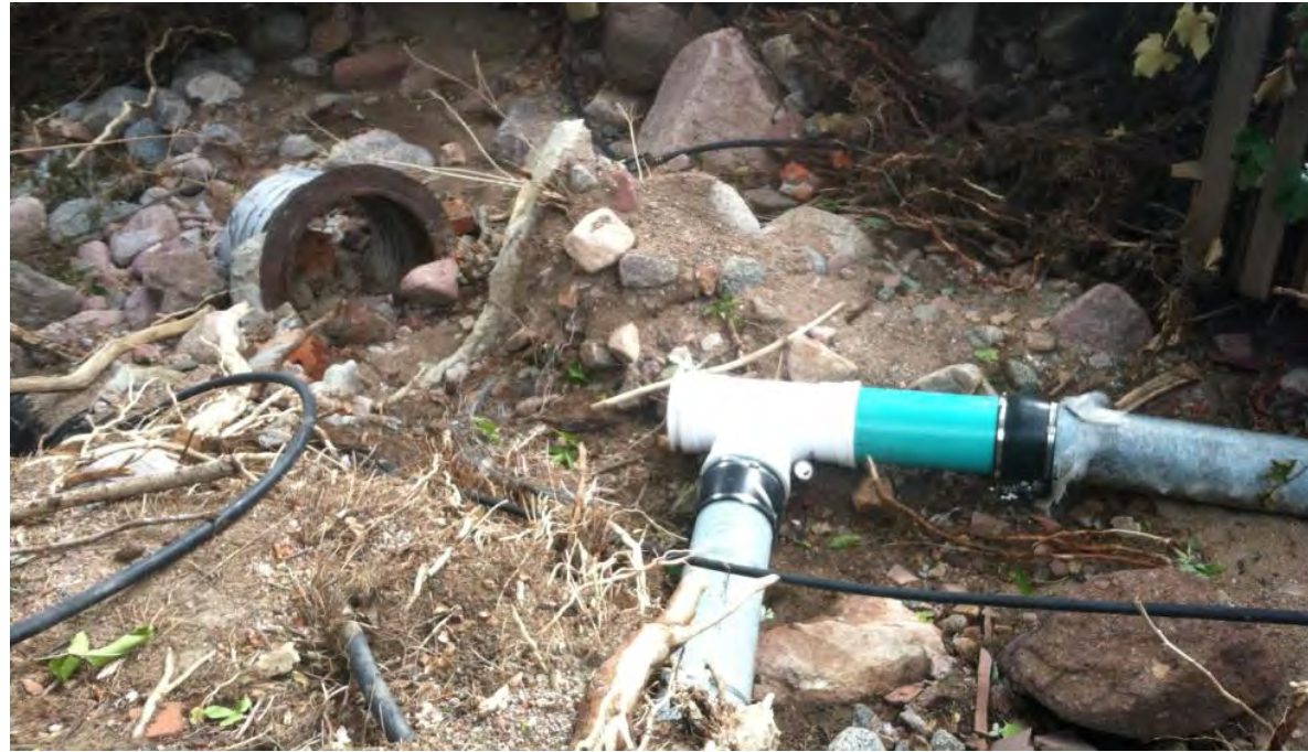
Sewer Manhole Damage - Sept. 2013
