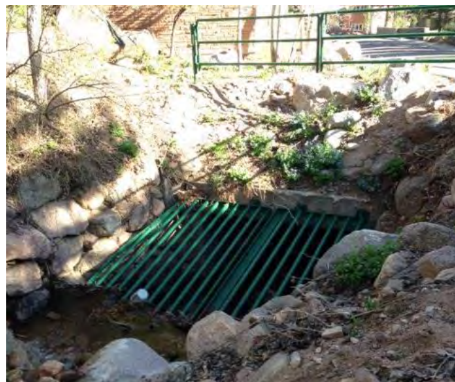
New Trash Rack
