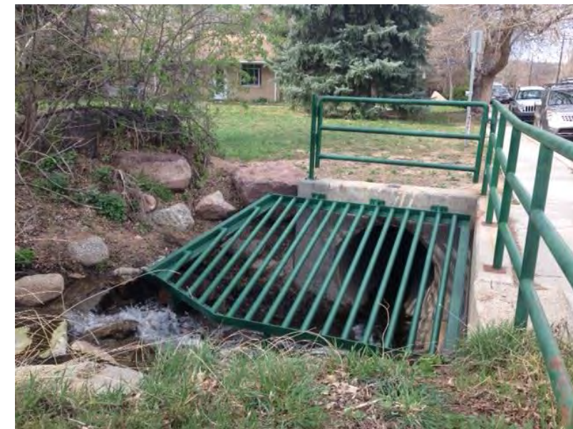
New Trash Rack
