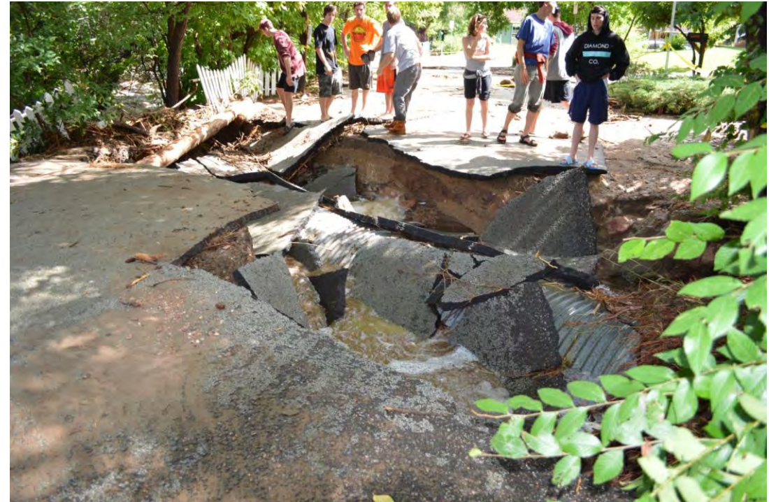
Sept. 2013 Flood Damage
