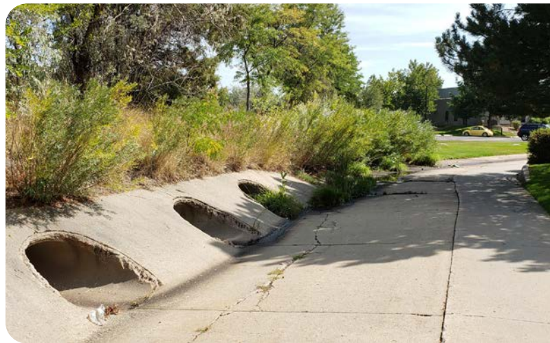
Flatirons Park Stormwater Drainage
