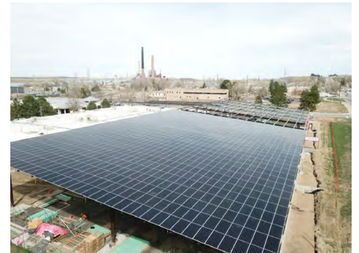
Avalon Ballroom's carport solar panel canopy, the largest in Boulder County. Source: customsolar.us
