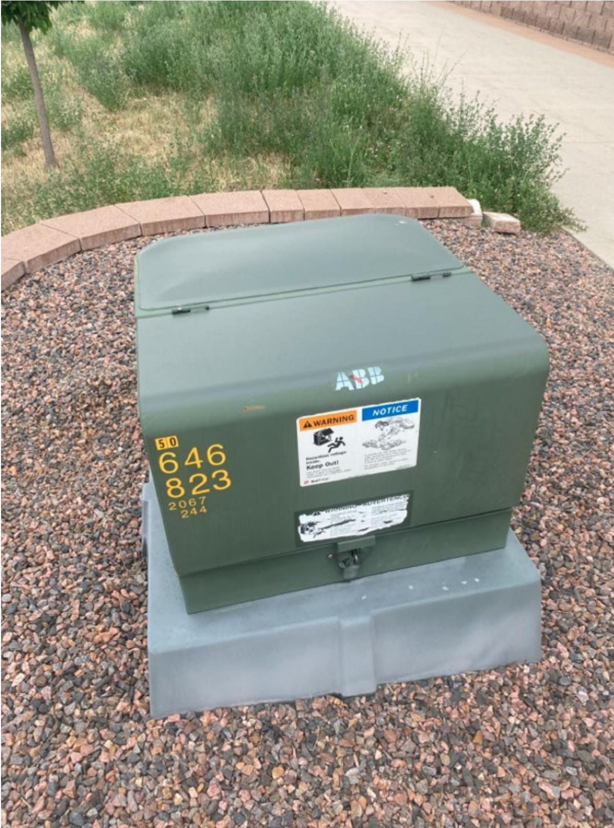
Padmount Transformer (50kVA typ.):
