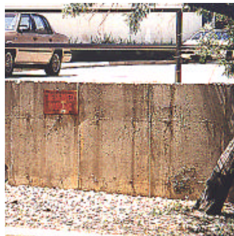
▲ 3.1.M. Avoid using blank concrete retaining walls to handle grade differences with abutting properties.
